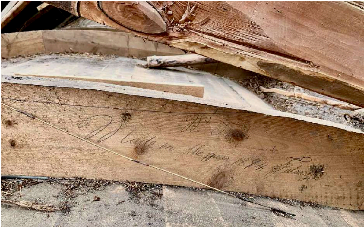
FIGURE 16C: Carpenter's signature on one of the saucer vault ribs record that the ceiling was added in 1894. This practice has been revived at Leipoldt House and other new joinery forming part of the restoration process. (Figure 10F). (Image: ARCON, 1 Nov. 2019).
