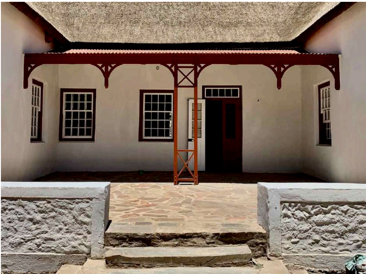
FIGURE 15F: Rear veranda of the Winkelhuis with reconstructed canopy based on a photograph that the author, by pure coincidence, took on a casual visit to Wupperthal about 4 months before the fire. That photograph proved to be the only known record of the rear façade of the house with its canopy. (Image: ARCON, 27 November 2020).
