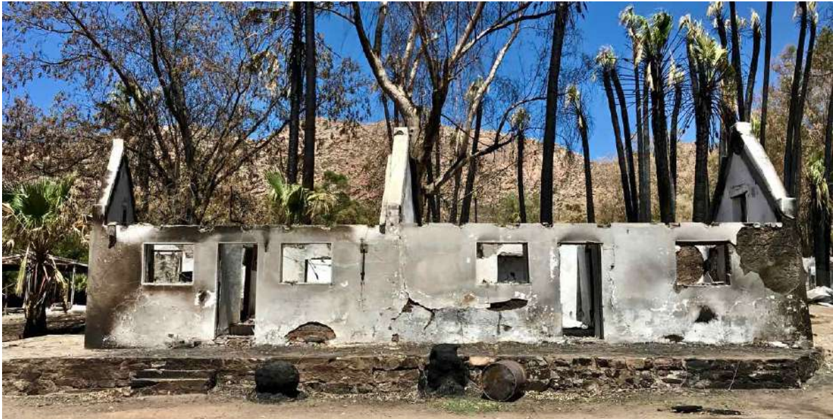
FIGURE 21A: The gutted Palms Guest House after the fire. (Image: ARCON, 24 January 2019).
