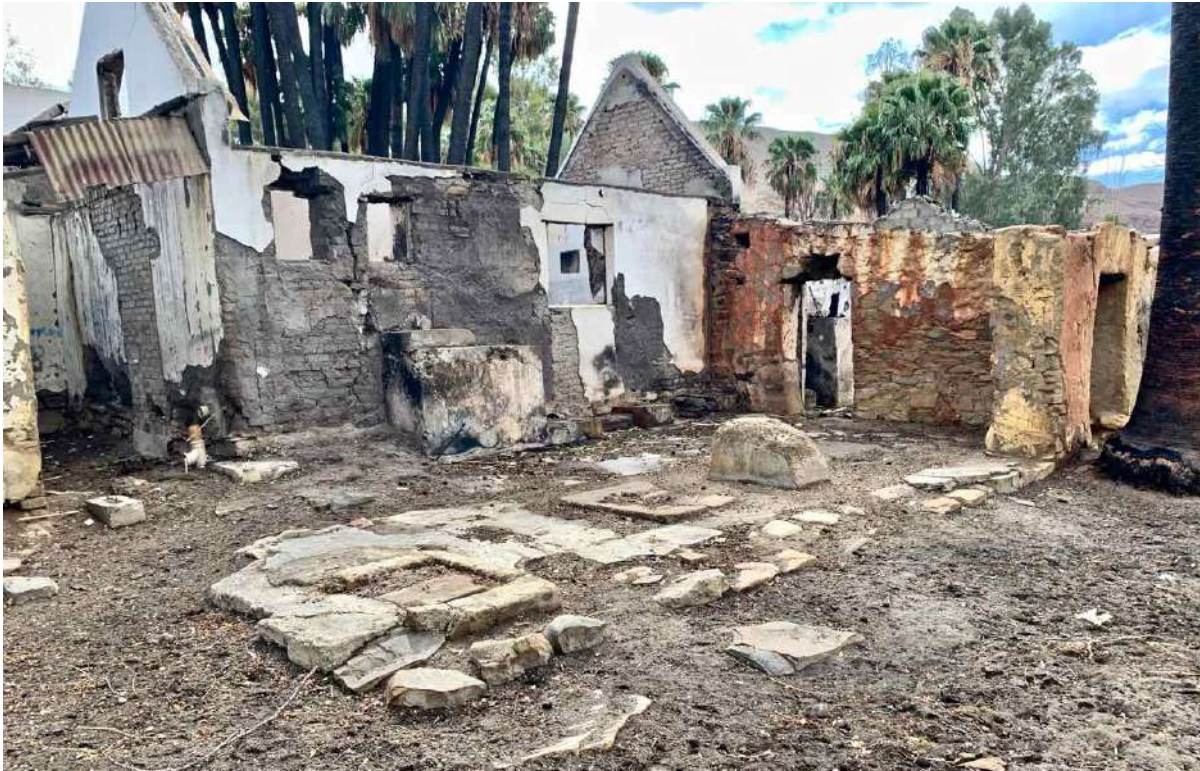
FIGURE 19D: View of the back of the tannery after the fire (southwest end) showing various remnants of cement and concrete bases which once supported tanning machinery. The 'stoep' in the foreground was once under a lean-to roof, and remains of an old stone wall base are visible running diagonally across the foreground (Image: ARCON, 6 December 2019).
