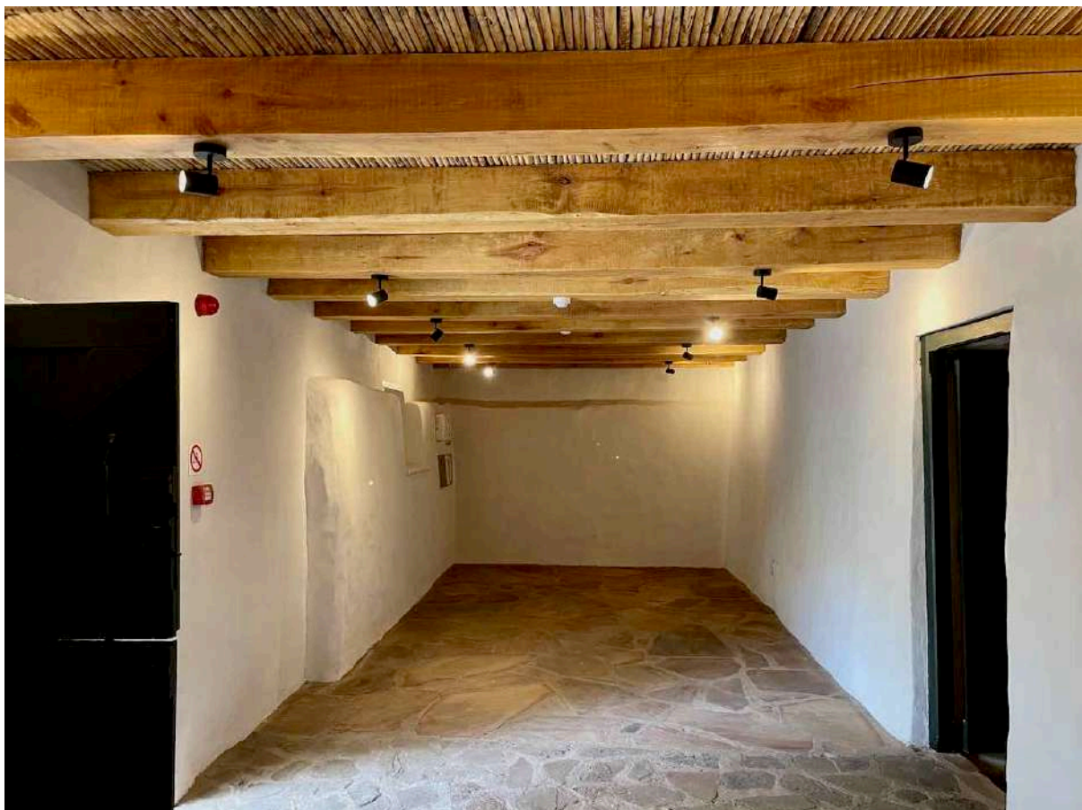
FIGURE 23F: New fire alarm system in Leipoldt House. The panic button and red alarm light are next to the front door (left) with the control panels at the left far end. Smoke detectors are mounted to the underside of new rafters supporting a new brandsolder and reed ceiling. (Images: ARCON, 8 June 2021).
