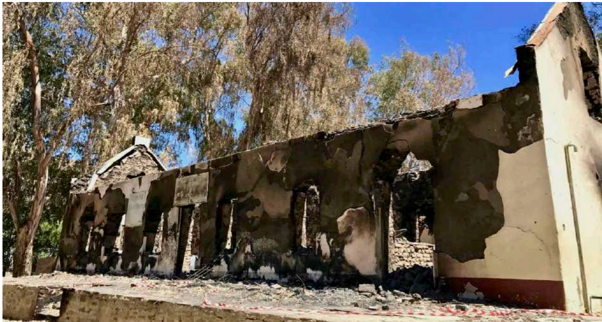
FIGURE 13A: The Mission Stores Building after the fire. (Image: ARCON, 24 January 2019).
