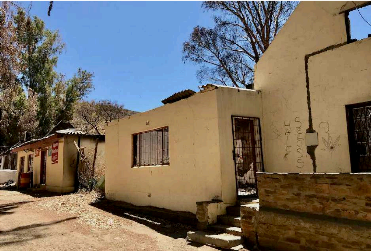
FIGURE 26B: The western end of the Mission Stores with flat roofed kitchen extension (center) and the derelict café building on the far left. (Image ARCON, 24 February 2019).
