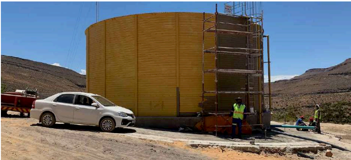
FIGURE 27A: The new reservoir funded by the Foundation nearing completion. (Image ARCON, 14 January 2021).
