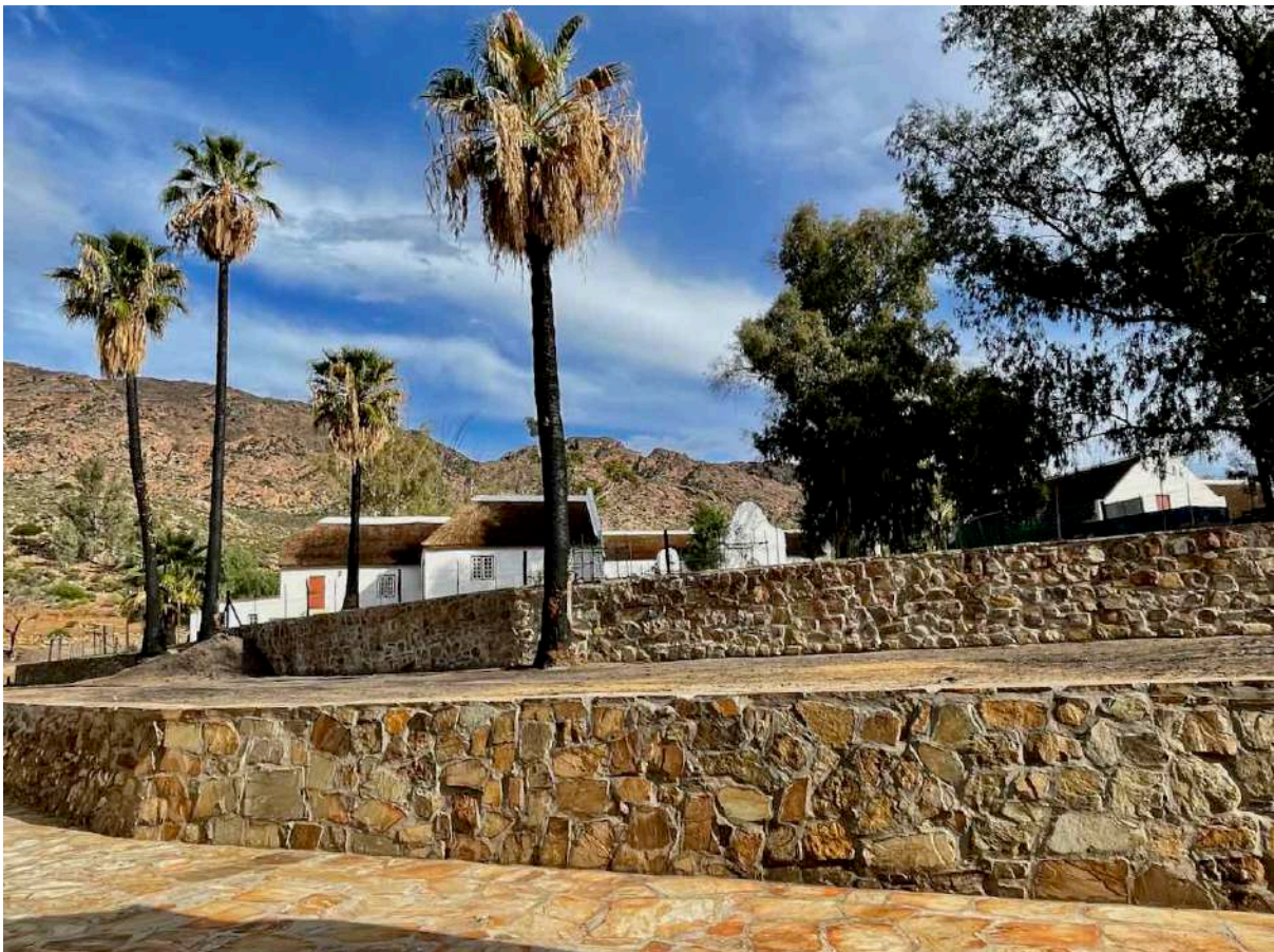
FIGURE 26E: The stone retaining walls after reconstruction behind the Hostel Buildings. (Image ARCON, 8 June 2021).
