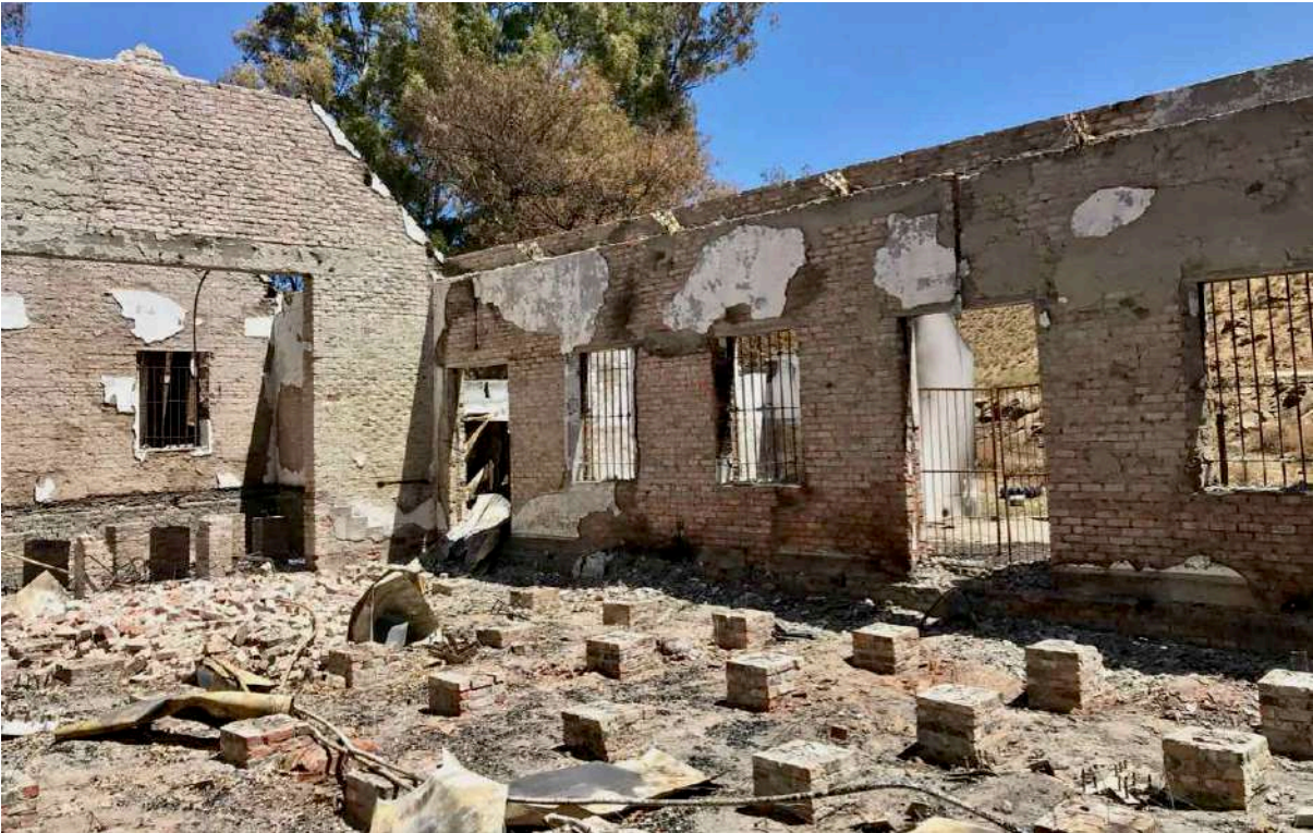
FIGURE 11C: Gutted interior of the Community Hall after the fire. (Image: ARCON, 24 January 2019).
