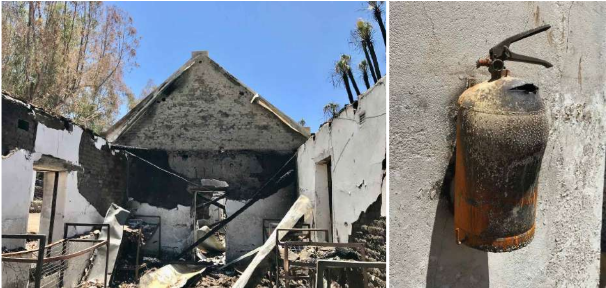
FIGURE 6: Left: One of the gutted school hostels littered with mangled bed frames and building debris. Right: The fire spread so rapidly that the fire extinguishers could not be used. This example was left to explode on its wall bracket. (Image: ARCON, 24 January 2019).
