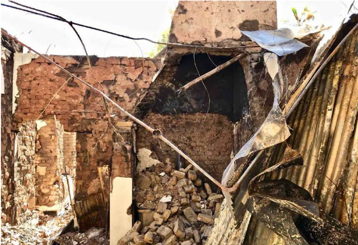
FIGURE 15E: Collapsed kitchen hearth in the Winkelhuis after the fire. All intact bricks were recovered and re-used in its reconstruction. (Image: ARCON, 24 January 2019).
