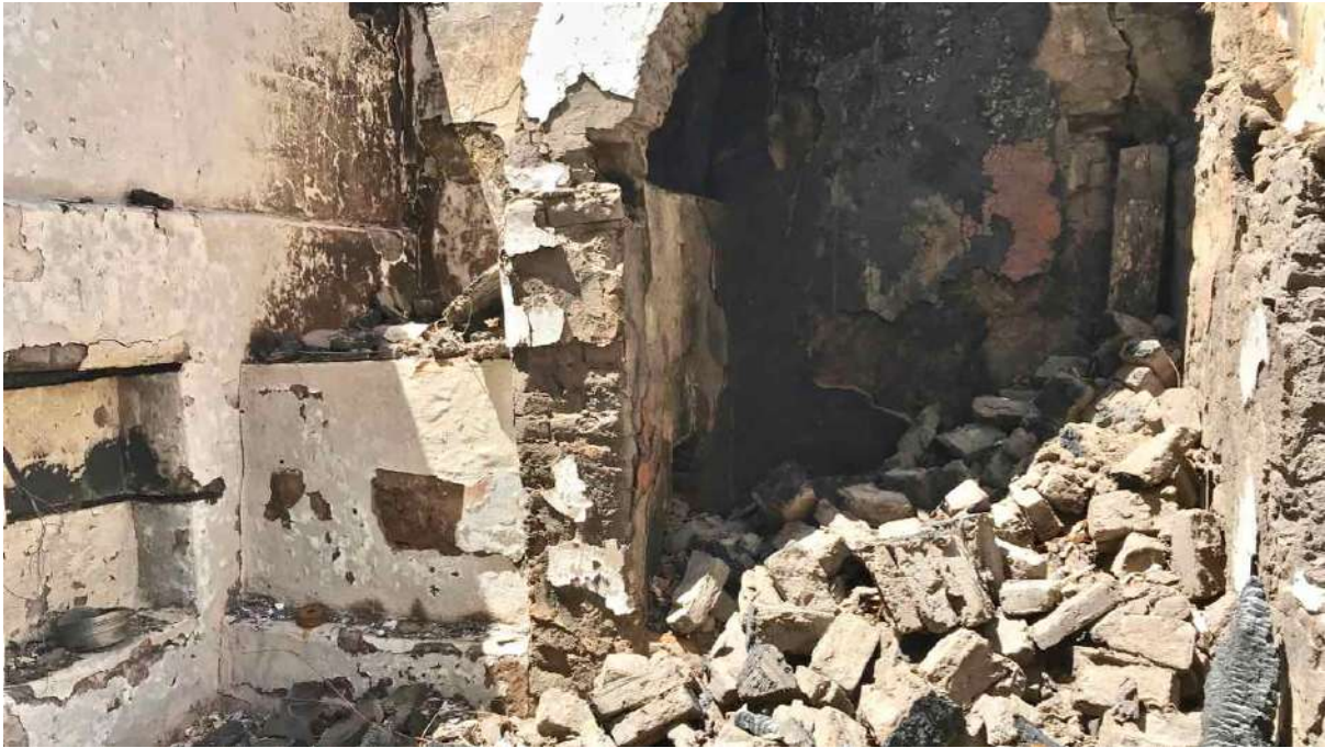
FIGURE 10C: The kitchen hearth of Leipoldt House after the fire which collapsed after the supporting bressumer beam burned through. (Image: ARCON, 24 January 2019).
