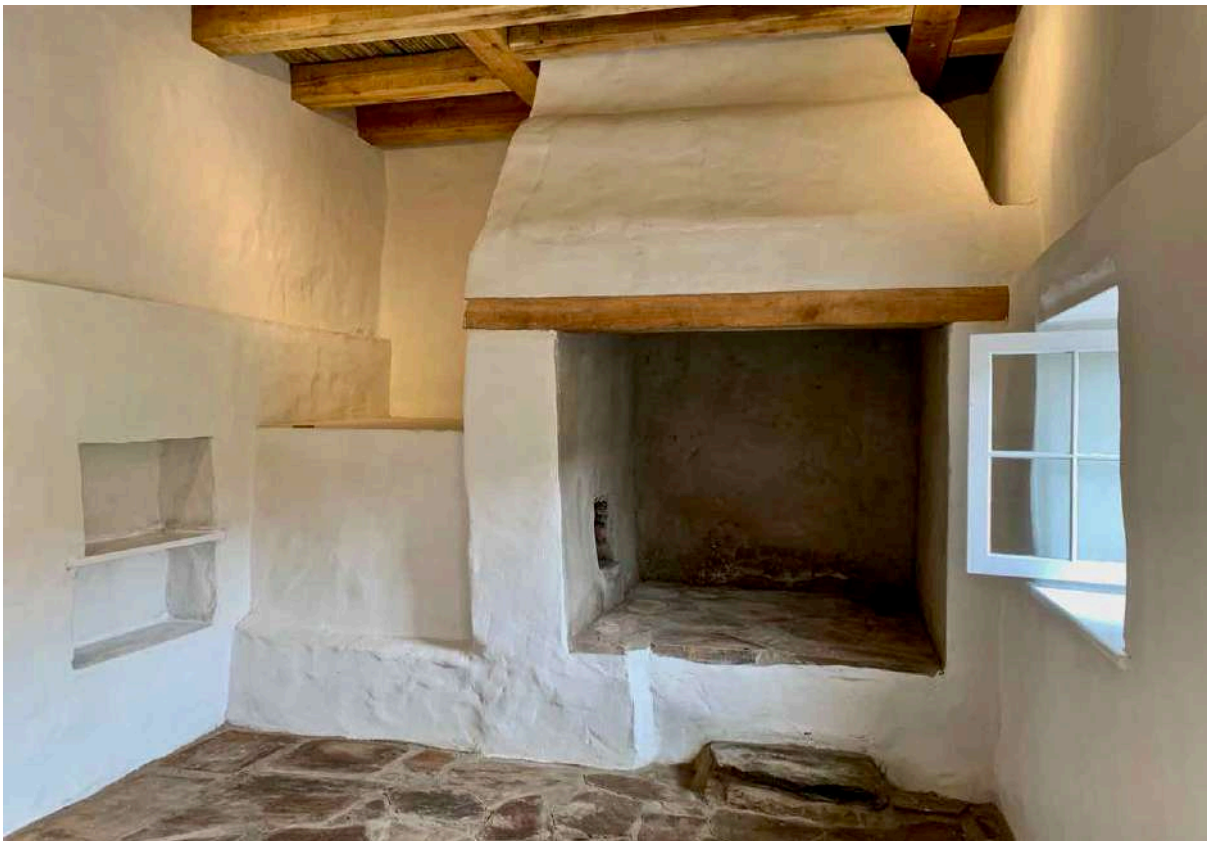
FIGURE 10D: The kitchen of Leipoldt House after restoration and reconstruction of the hearth flue. (Image: ARCON, 1 September 2020).
