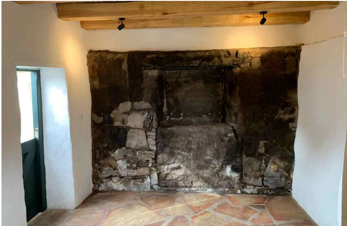
FIGURE 10E: Leipoldt House memorial wall: It was decided that one of the end walls in Leipoldt House should be retained in the condition in which it was found after the fire to commemorate the disaster. This was considered especially relevant as this part of the building is scheduled to become the town's museum. (Image: ARCON, 8 June 2021).
