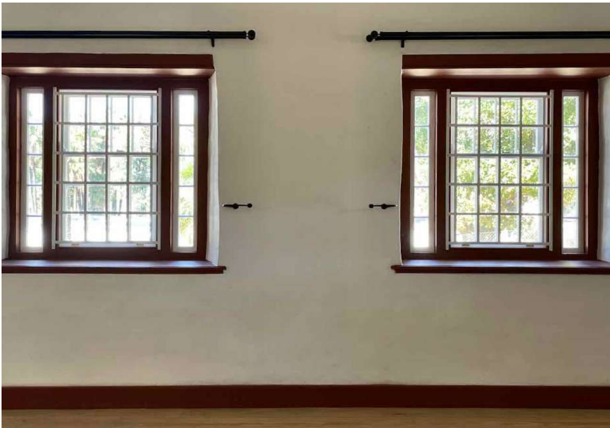
FIGURE 13F: Replacement windows in the Mission Stores after restoration. It is suspected that the additional glazing on the sides was to provide extra light for pupils when the building was still a school in the 1830's. (Image: ARCON, 7 April 2021).
