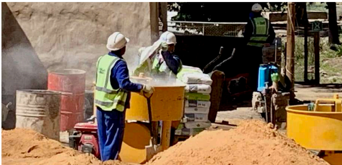
FIGURE 9: Pan mixers in action preparing lime/sand mortars and renders. The sand used was Malmesbury sand which is coarser and therefore preferred over finer Cape Flats silica sands for work on historic buildings. (Image: ARCON, 25 October 2019).
