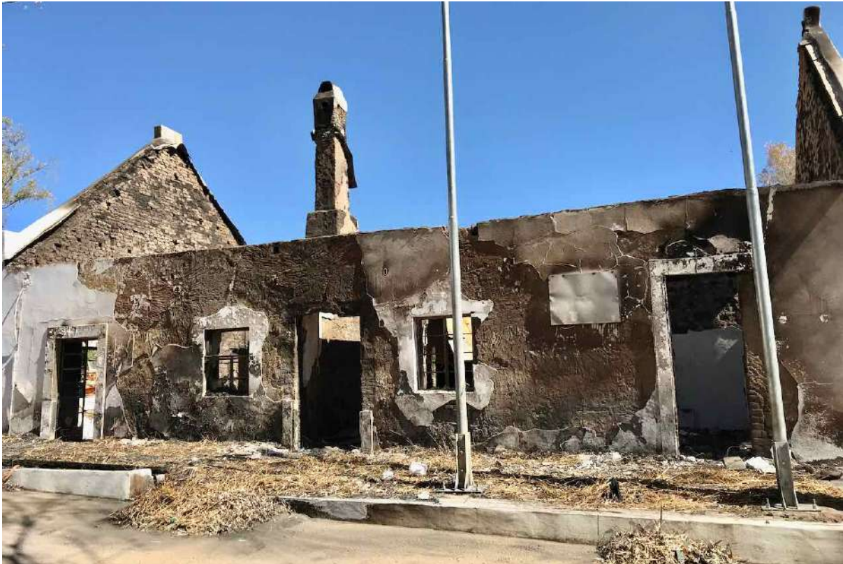
FIGURE 4: The fire gutted 'Winkelhuis' (Shopkeeper's House) after the fire. The building had been the administration headquarters for the town before the fire. This image is typical of the degree of damage sustained. (Image: ARCON, 24 January 2019).
