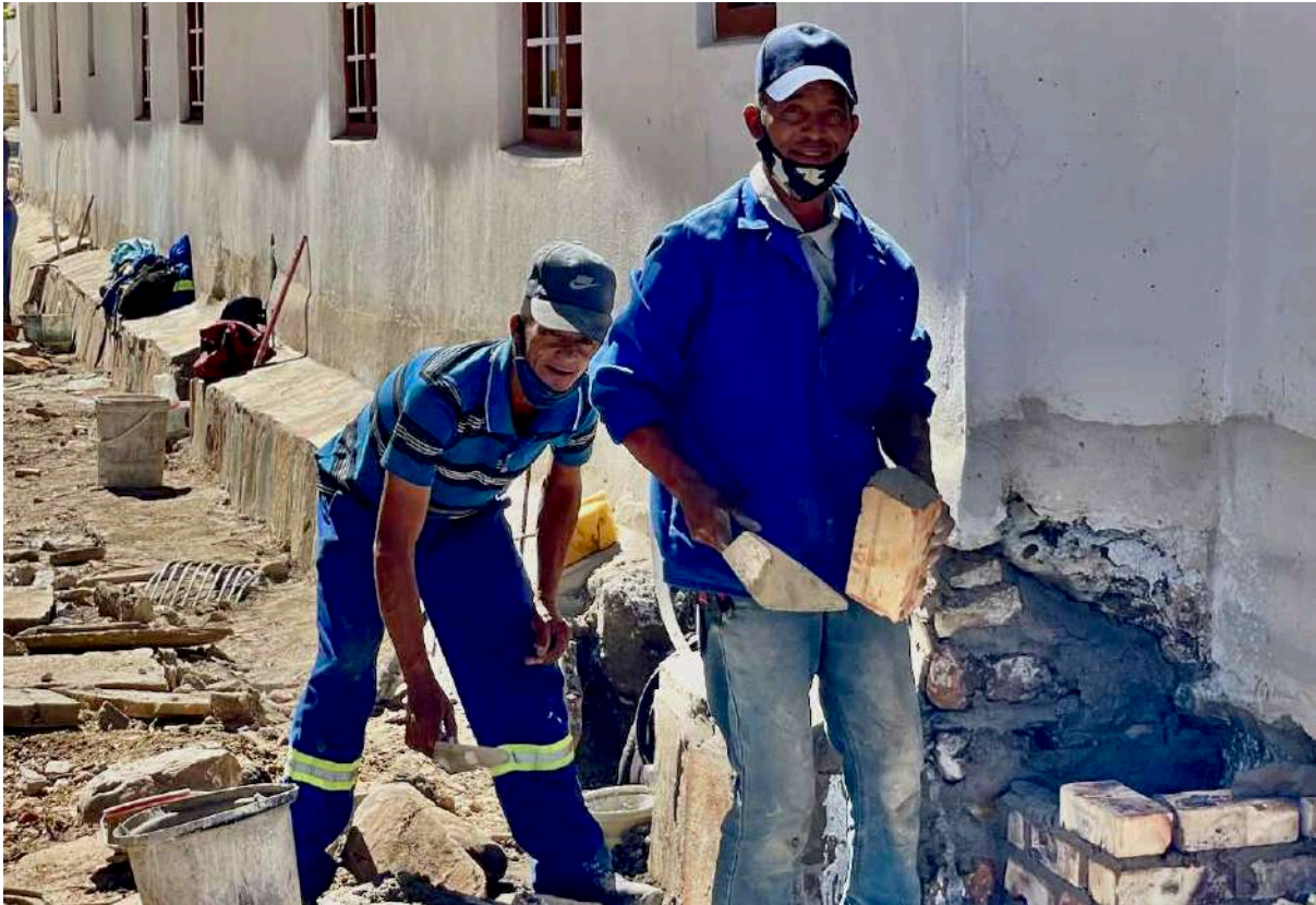
7 April 2021: Wall repairs at the back of one of the School Hostel buildings.
