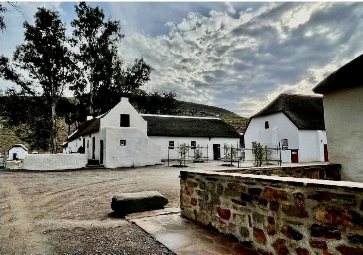
FIGURE 26C: The same view but with the kitchen extension and derelict café now removed, reclaiming the open space between the mission Stores and Leipoldt House. (Image ARCON, 8 June 2021).
