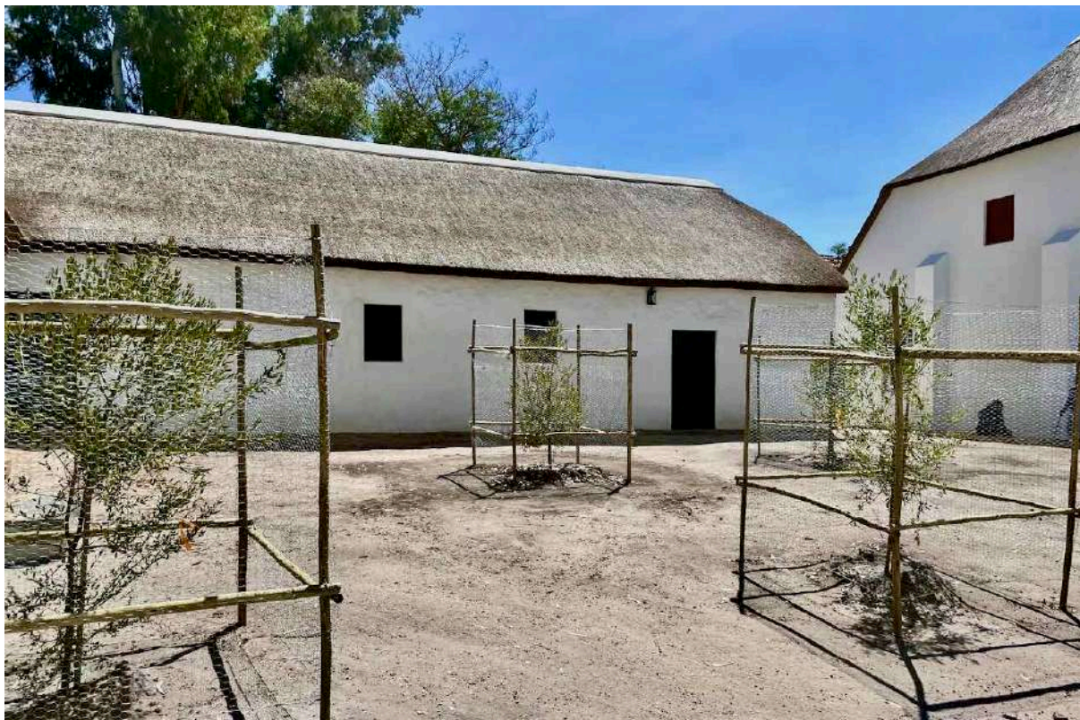
FIGURE 26A: Simple new landscaping in the reclaimed open space after the demolition of a derelict café building between Leipoldt House and the Mission Stores. The tree enclosures comprise hand cut local laths and diamond mesh fencing to keep wandering donkeys at bay. The rear wing of Leipoldt House is in the background. (Image ARCON, 27 October 2020).
