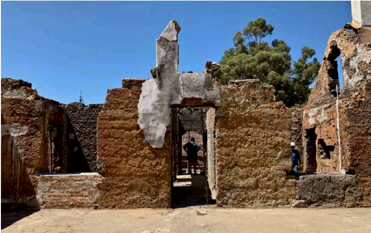
FIGURE 14C: The front façade of the Parsonage after the fire debris had been cleared. The rammed earth construction of the central portion of the facade is clearly evident in the horizontal wall striations. (Image: ARCON, 30 January 2020).
