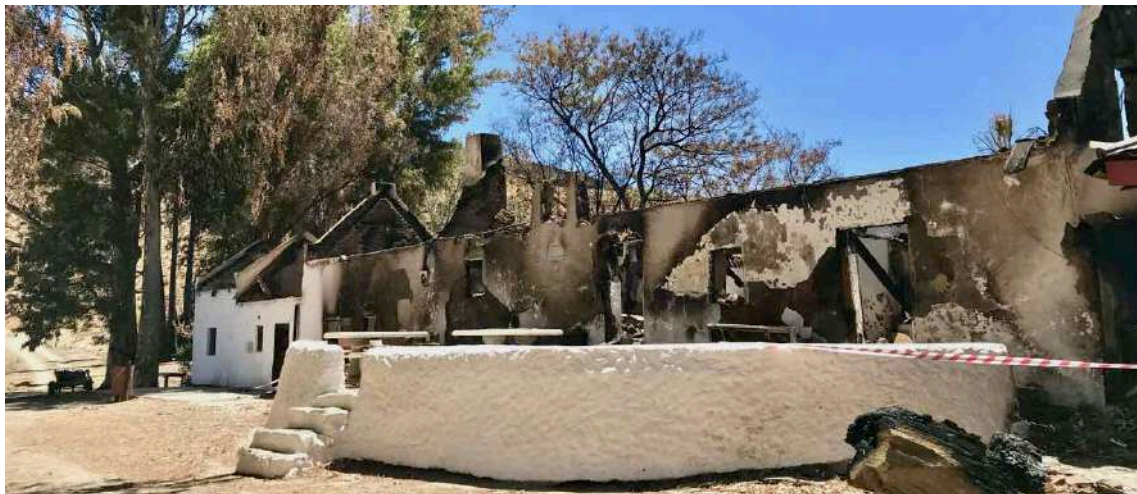
FIGURE 10A: Exterior of Leipoldt House after the fire. This building is most probably the original Rietmond farmhouse, pre-dating the arrival of the Rhenish missionaries by about 30 years. The uncharacteristic semicircular stoep appears to have been used as a podium from which open air services were conducted before the church was completed, explaining its non-traditional shape. (Image: ARCON, 25 October 2019).
