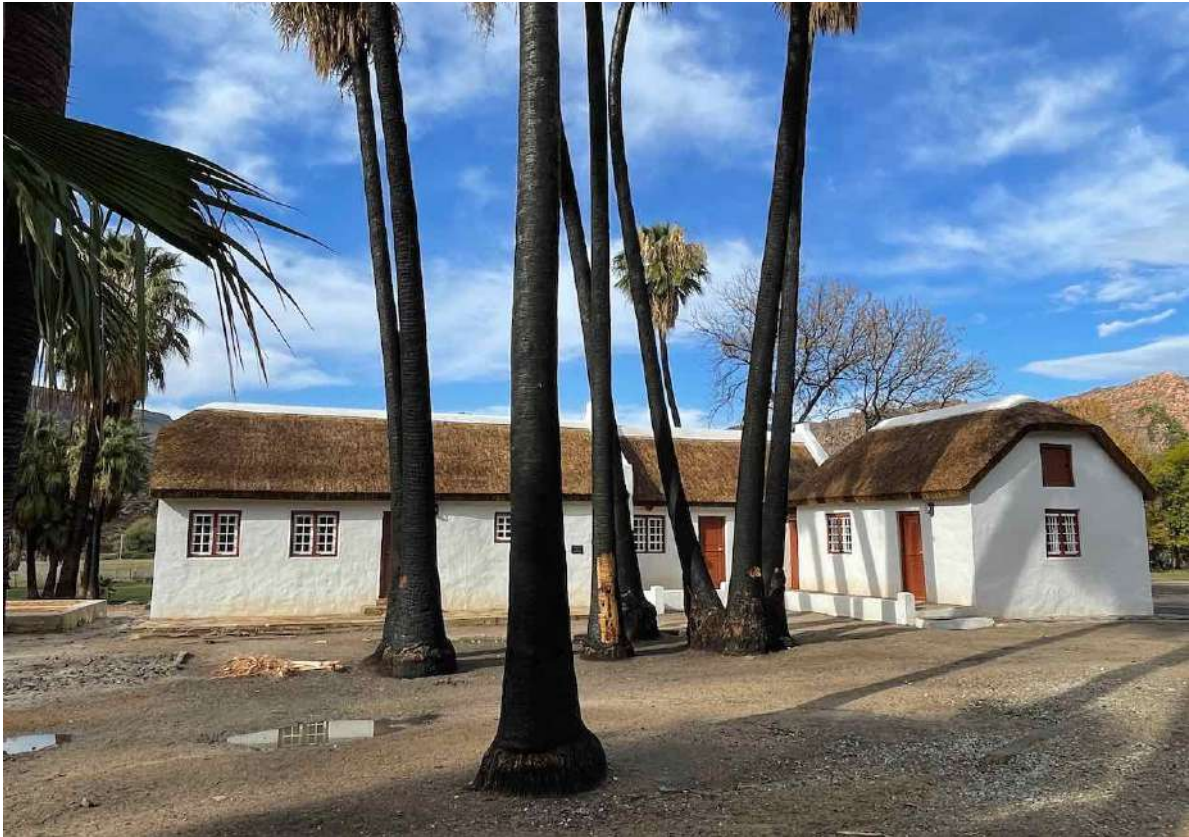
FIGURE 19B: The Old Tannery after restoration/reconstruction. Part of one of the old tanning tanks is just visible in line with the building on the extreme left. (Image: ARCON 4 May 2021).
