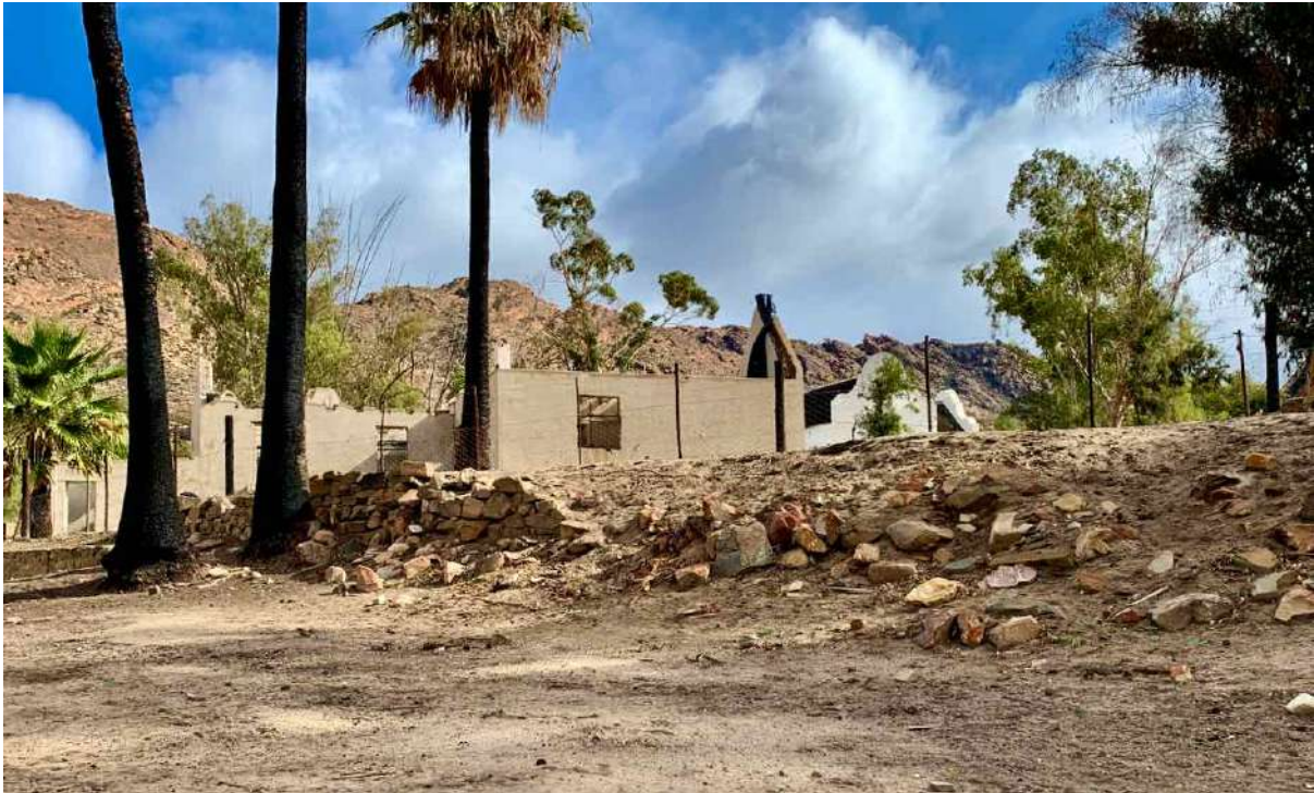
FIGURE 26D: The stone retaining wall in very poor condition behind the Hostel Buildings. The Old Parsonage is left of center with the Church to the right of center beyond. (Image ARCON, 26 May 2020).
