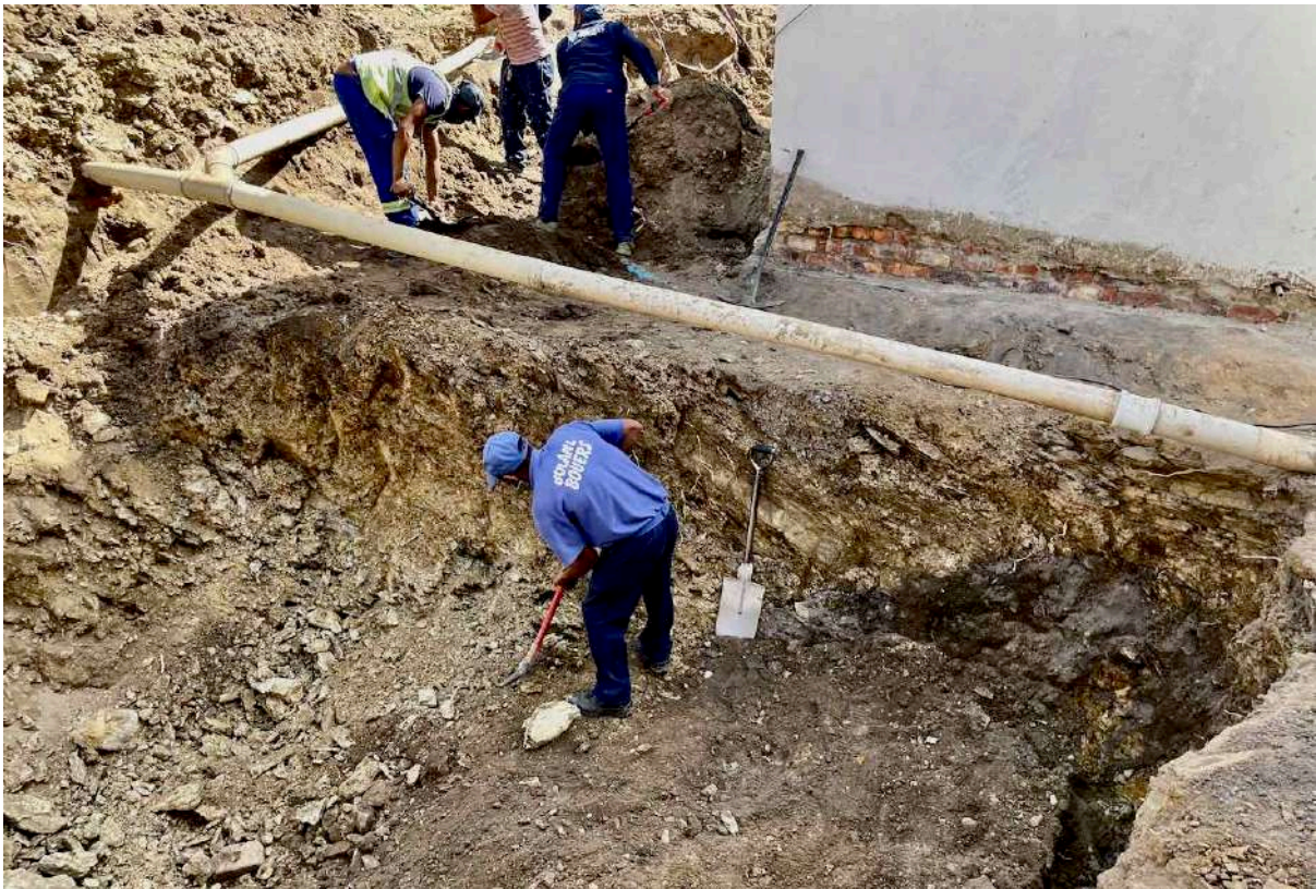
9 March 2021: Digging the massive new underground stormwater sump behind the School Hostels
