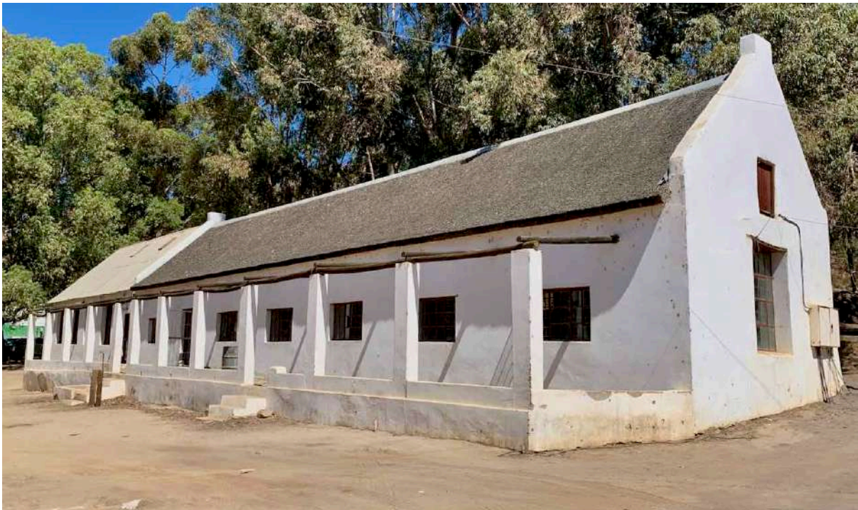
FIGURE 18D: Exterior of the shoe factory prior to refurbishment. It had been re-thatched by the Moravian Church a few years previously. The extension on the far left was then used as the town library and had a corrugated iron roof. (Image: ARCON, 17 March 2020).
