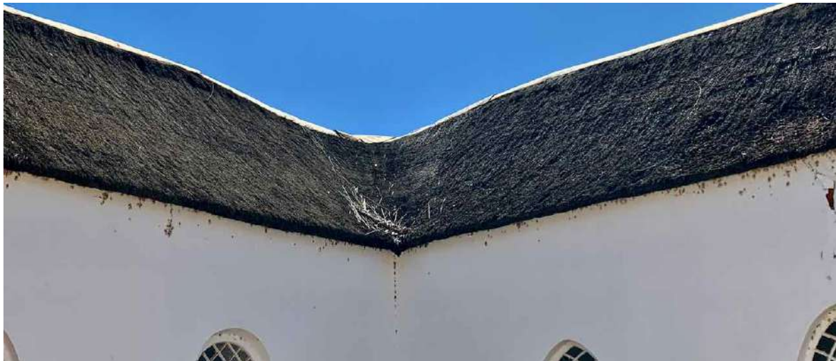
FIGURE 16A: View of the thatch roof of the church before reconstruction. The roof was in very poor condition and in a state of near collapse between nave and transept. (Image: ARCON, 1 Nov. 2019).
