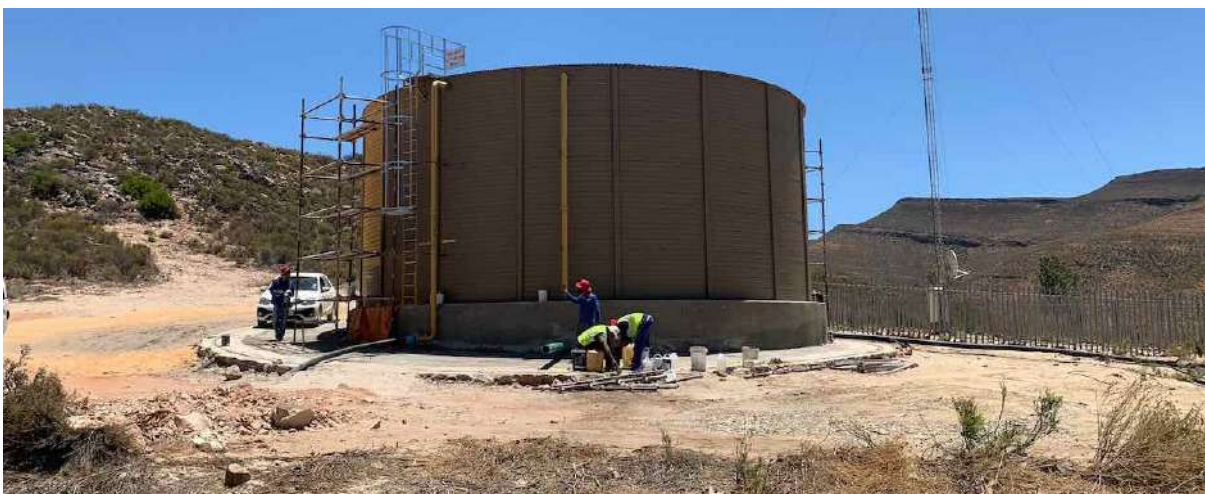
FIGURE 27B: The new reservoir painted to match the surrounding mountainsides but is in any case largely obscured from the Church Precinct below. (Image ARCON, 14 January 2021).
