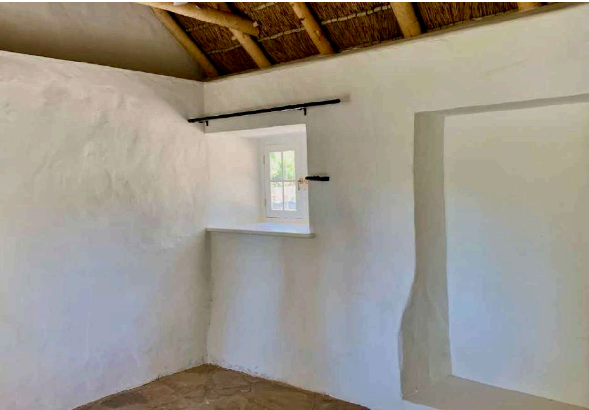
FIGURE 21D: The same part of the interior after restoration. (Image: ARCON, 10 November 2020).
