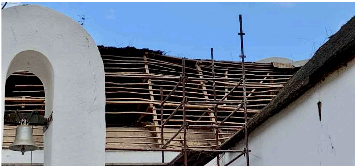
FIGURE 16B: The roof with thatch removed showing the very poor condition of the roof timbers. (Image: ARCON, 1 Nov. 2019).
