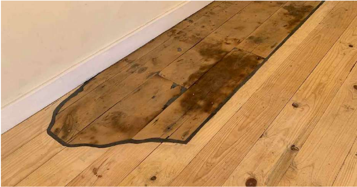
FIGURE 15E: Remnant of cedarwood flooring recovered after the fire and set into the new floor in the same position where it had been recovered. An interpretative plaque explaining the significance of these floorboards has been placed on the wall above. Out of all the buildings damaged in the fire, this is the only area where some cedarwood flooring survived. (Image: ARCON, 27 November 2020).
