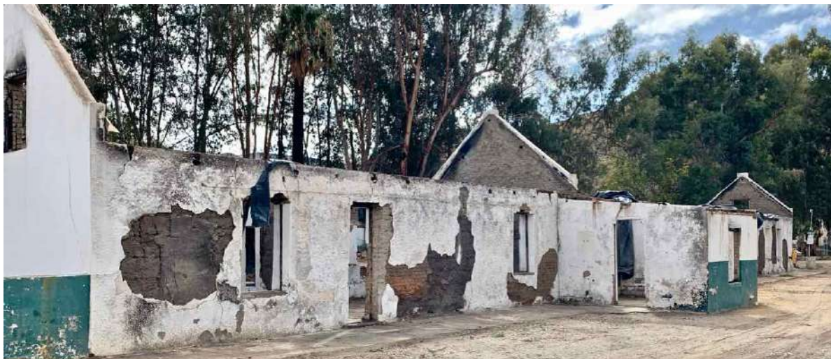
FIGURE 20A: The northernmost of the two school hostels after the fire. (Image: ARCON, 24 January 2019).
