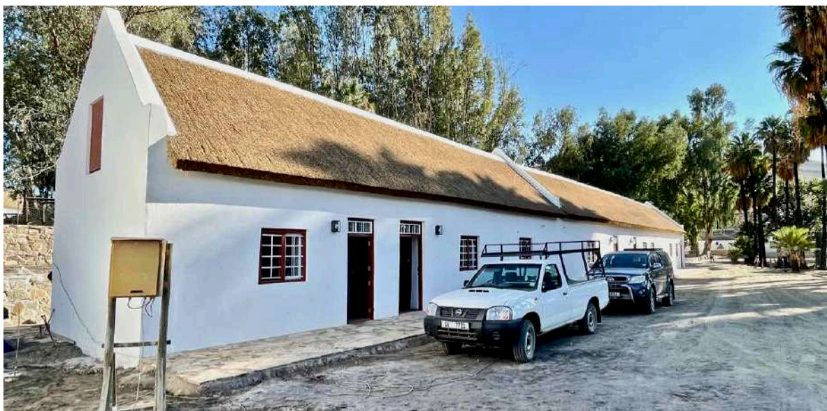
FIGURE 20B: The northernmost of the two school hostels with restoration nearing completion. New casement windows were installed in the openings of the burned out 20 th C false sash windows which had, in turn, probably replaced the original windows, possibly similar to the surviving casement windows in the Shoe Factory ( Figure 17A ) except that the latter are single casements and not double casements as installed here. (Image: ARCON, 4 May 2021).
