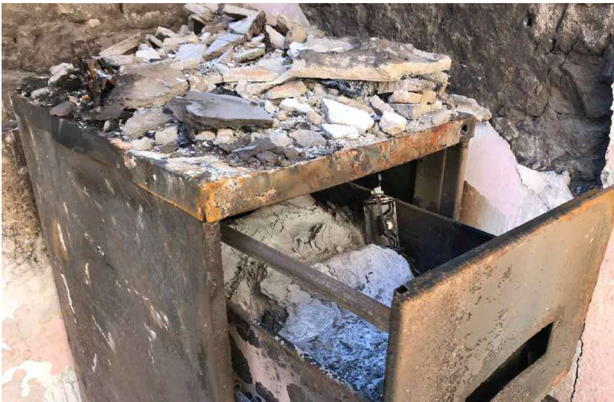
FIGURE 5: Most of the town's records were lost in the fire. That included drawings, photographs, title deeds, survey diagrams and other historic and historical records that would otherwise have been useful for informing the reconstruction process. (Image: ARCON, 24 January 2019).
