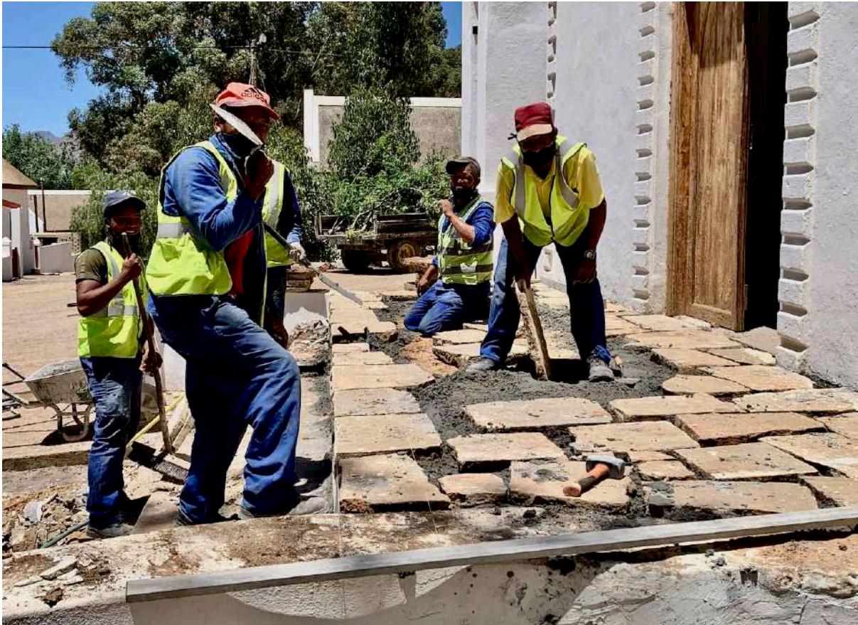
FIGURE 16E: Workers re-laying the stone flags in front of the church. The grey mortar is lime mixed with local dark grey river sand and not cement. (Image: ARCON, 27 November 2020).
