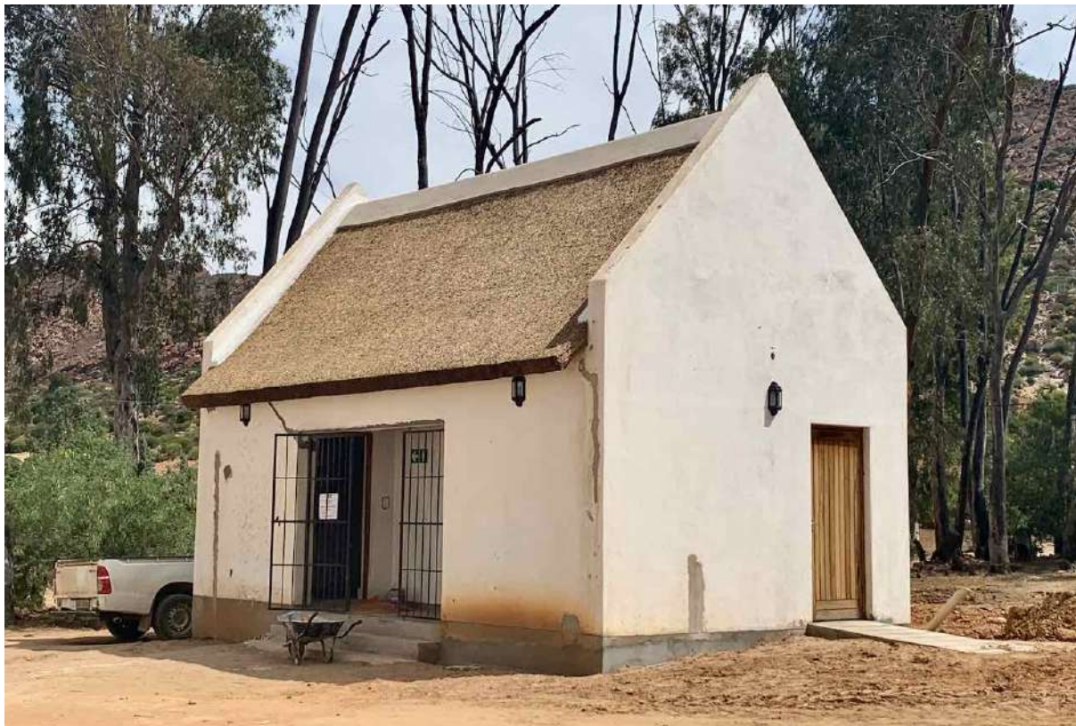
FIGURE 24B: The church ablution after re-thatching and undergoing crack repairs prior to repainting. (Image ARCON, 27 October 2020).
