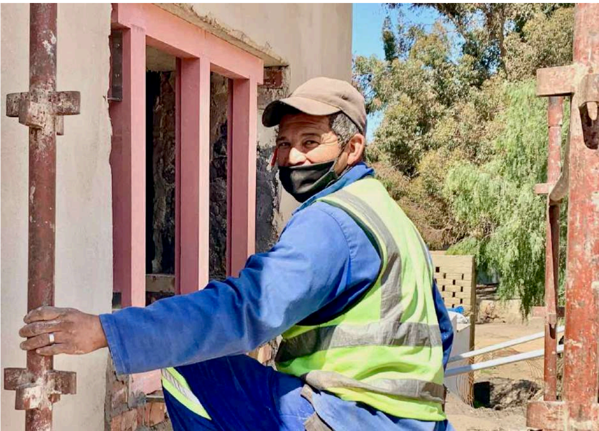
16 September 2020: Fitting one of the new window frames at the Old Parsonage.
