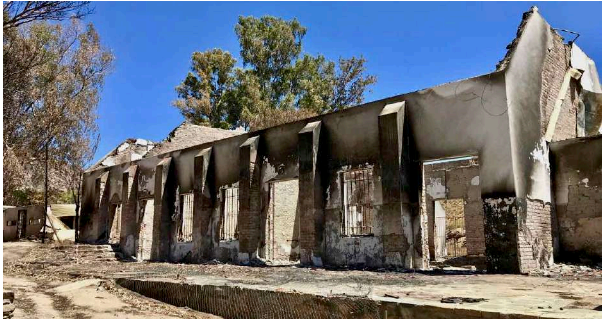
FIGURE 11A: Exterior of the Community Hall after the fire. (Image: ARCON, 24 January 2019).
