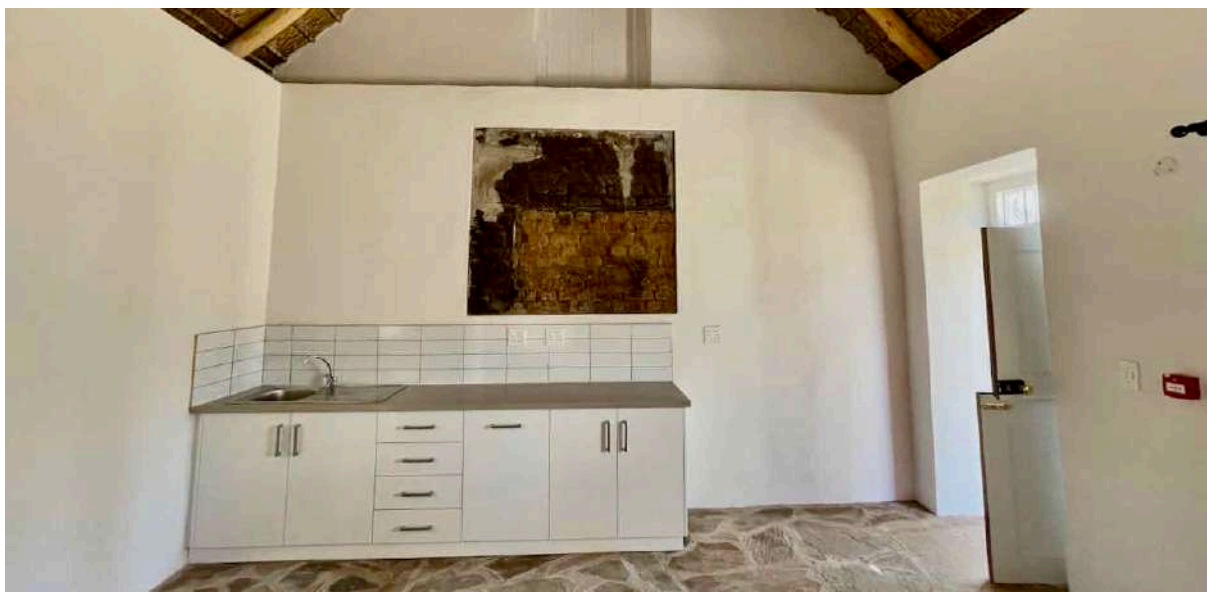
FIGURE 28B: Masonry panel left un-plastered and treated with a special breathable fixative to prevent it from dusting. This panel shows three periods of construction with a partly charred lintel from the fire still in place. This image was taken before the interpretive plaque was fixed to the wall. (Image ARCON, 14 January 2021).
