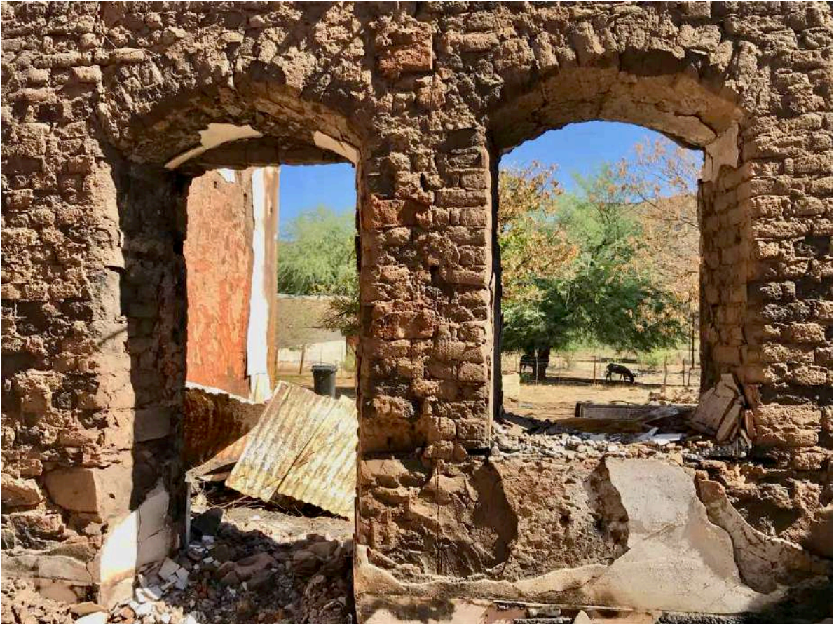
FIGURE 15C: From the lounge interior of the Winkelhuis looking through to the back garden after the fire. (Image: ARCON, 24 January 2019).
