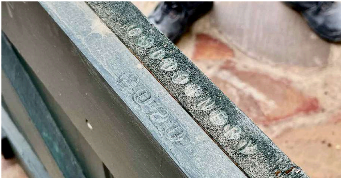
FIGURE 10F: Carpenter's marks: All new joinery in Leipoldt House and other buildings was stamped with the name of the joiner and date of fabrication in inconspicuous places as a record for future researchers: all in the tradition of historic carpenter's marks incised into their work through the ages, and consistent with similar early practices in the town (see Figure 16C ) (Image: ARCON, 8 June 2021).
