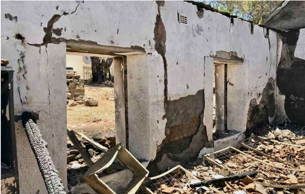
FIGURE 20C: Part of one of the hostel interiors shortly after the fire. The twisted remains of beds lie amongst the wreckage. (Image: ARCON, 24 January 2019).
