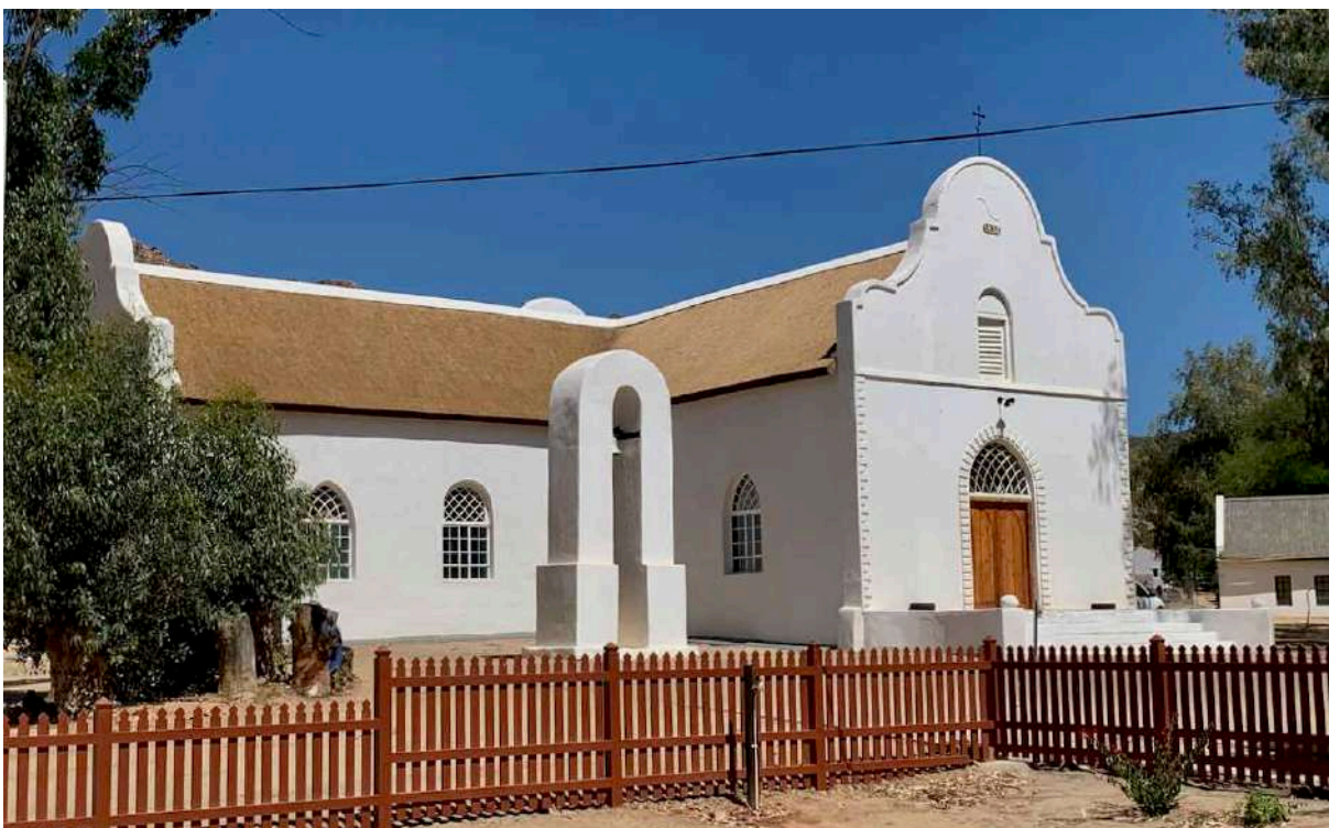
FIGURE 16F: The church building after completion of the new roof and repainting with a propriety breathable wall coating. (Image: ARCON, 14 January 2021).
