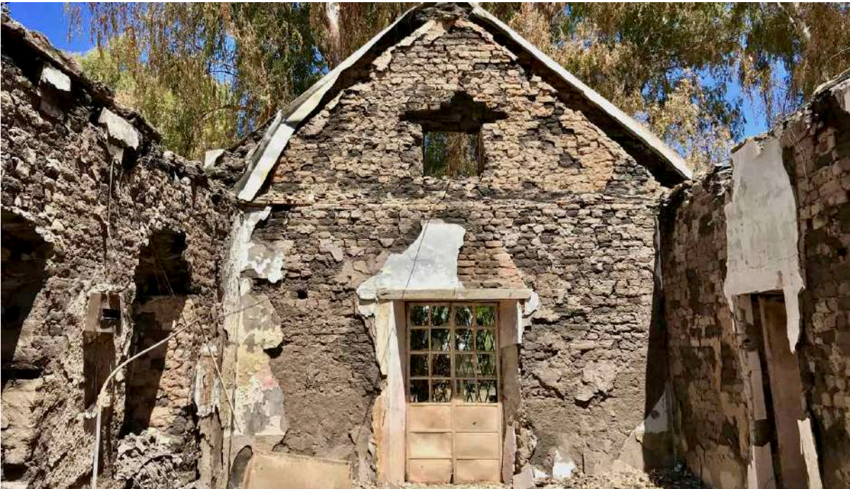
FIGURE 13C: Part of the Mission Stores interior after the fire. (Image: ARCON, 9 March 2021).
