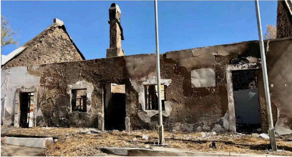
FIGURE 15A: The front façade of the Winkelhuis after the fire. This was one of the buildings initially considered particularly dangerous with various large wall cracks. However, on closer examination, it was found that the cracks pre-dated the fire. (Image: ARCON, 23 March 2021).
