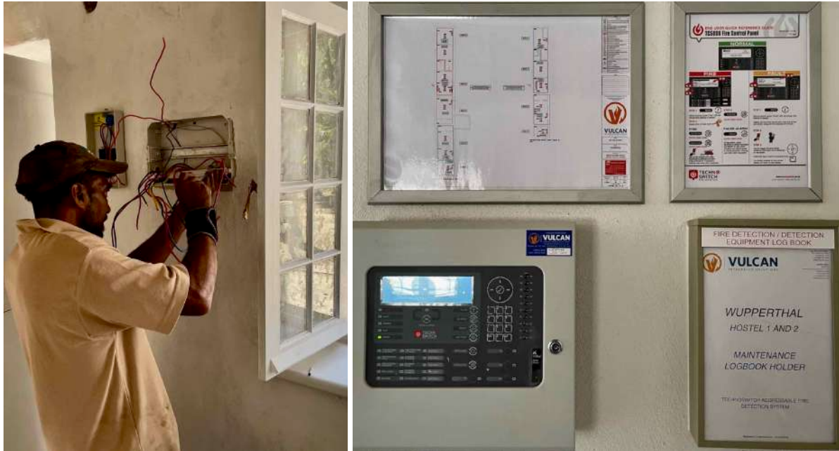
FIGURE 23E: New fire sensor and alarm systems were installed in all of the restored buildings. Prior to the fire, the only alarm system in the settlement had been the church bell. (Images: ARCON, 7 April 2021).
