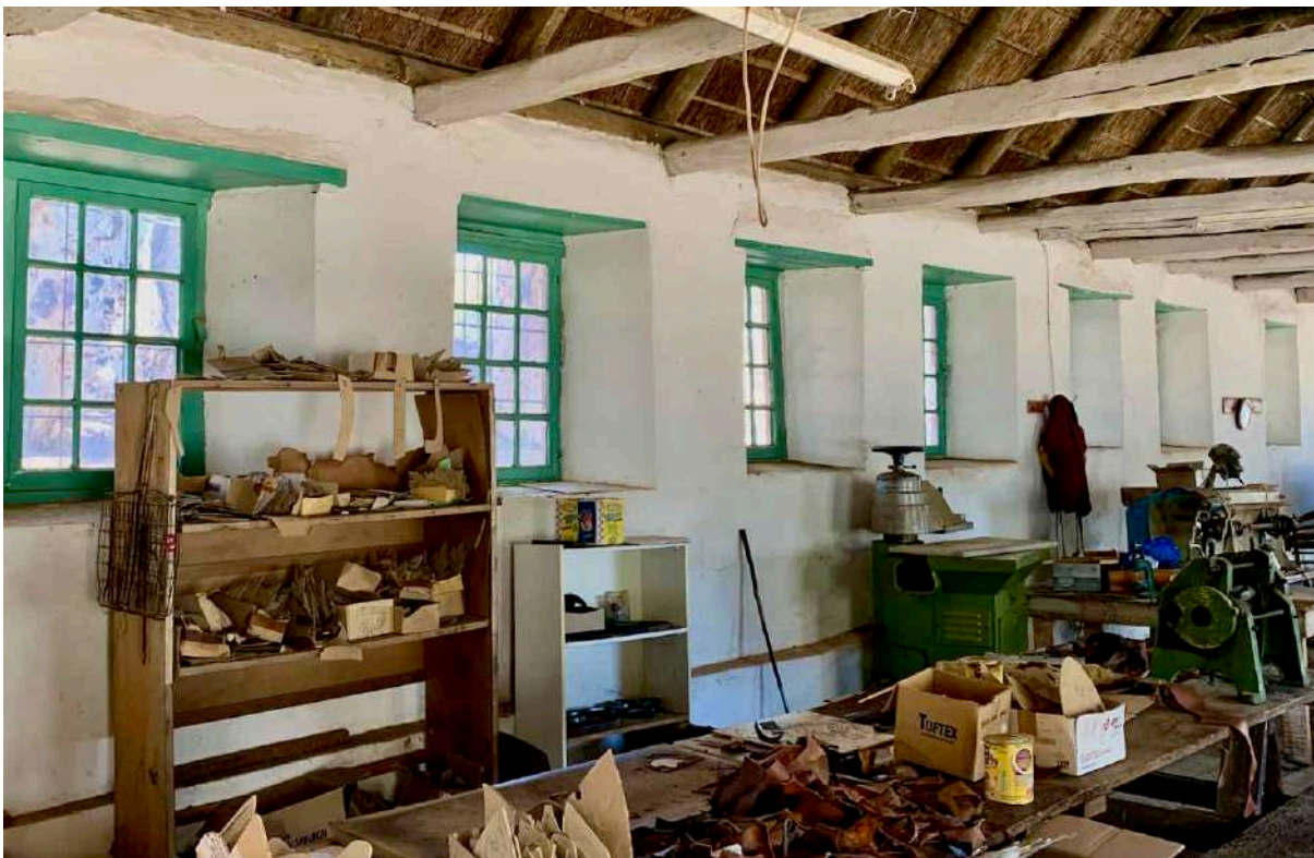
FIGURE 18A: Interior of the Shoe Factory before refurbishment with surviving original casement windows; now in all likelihood the oldest surviving casement windows in the settlement since the fire. (Image: ARCON, 17 March 2020).
