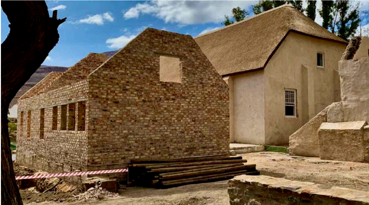
FIGURE 12A: The Creche Building under reconstruction (left) to accommodate new toilets and office space for the Community Hall. (Image: ARCON, 21 January 2020).
