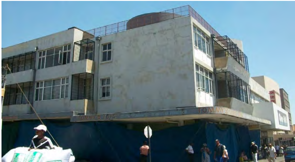
Fig. 226 Mixed use corner building on Kenilworth side border of Rosettenville (Source: tsica heritage consultants, 2015)
