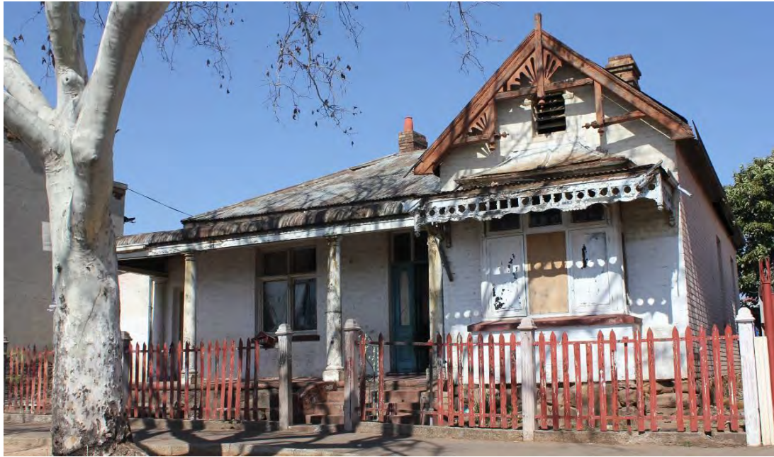
Fig. 160 Front façade showing the bad state of repair (Source: tsica heritage consultants, 2015)
