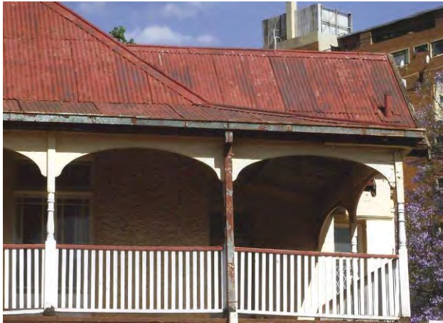
Fig. 23 Park Lane_Victorian colonial residence with perimeter verandah and steep corrugated iron roofing. Once a prominent double storey landmark off the old wagon road to Pretoria, via Halfway House (Photograph: Clive Chipkin)
