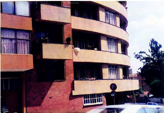
Fig. 29 Royal Crescent (right) on the curve; Reading Court (left) which is a major example of a Modern Movement building, restoration work is needed (Photograph: Clive Chipkin)
