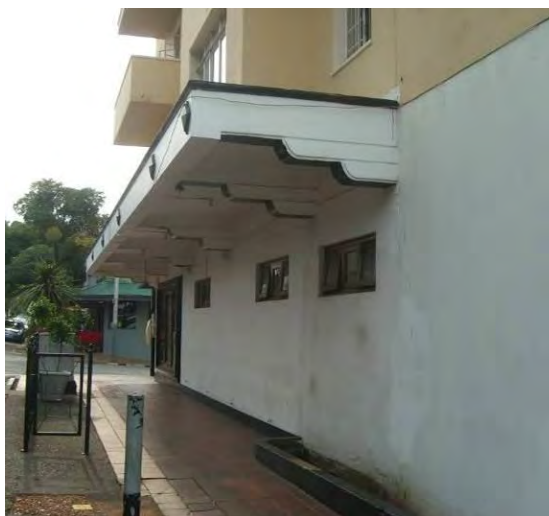
Fig. 6 Melville Mansions, 7 th Street in Melville_example for reinforced concrete cantilever, for Art Deco buildings slabs were supported on brackets with stepped or rounded edge forms.
