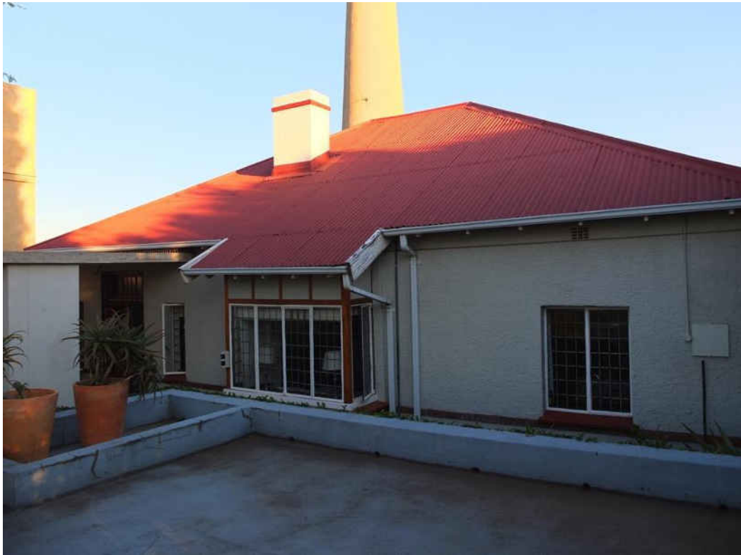
Fig. 263 Corrugated iron roof with side gables and central veranda, north elevation (Source: tsica heritage consultants, 2016)
