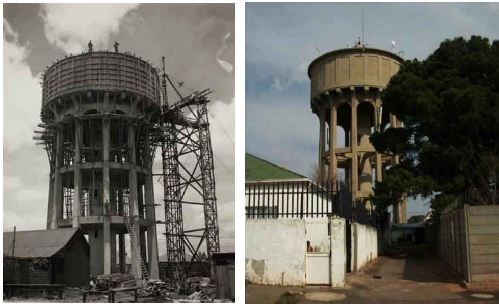
Fig. 287 & Fig. 288 On the left, the Brixton tower under construction in 1939 and on the right as it looks today (Source: Museum Africa and tsica heritage consultants, 2015)
