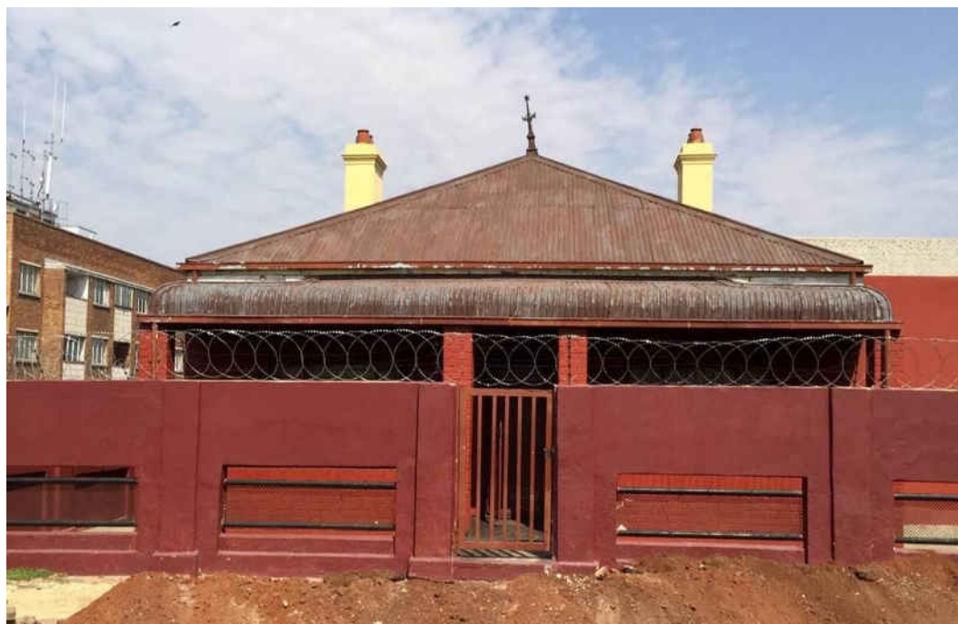
Fig. 142 Corrugated iron roof single storey house with two double chimneys and pots (Source: tsica heritage consultants, 2015)
